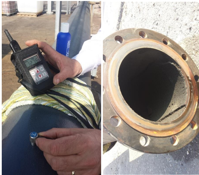
Figure 6.7 Manual wall thickness measurement and disconnected piece of horizontal pipe between producer wellhead and separator (shown sideways), indicating 6mm of scale. Photo courtesy Martin van der Hout (DAGO).
